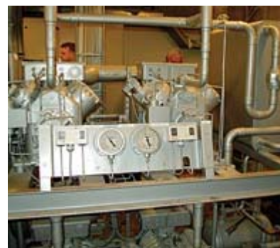
The Bitzer R-404A compressors are pictured here. There are two complete systems.
